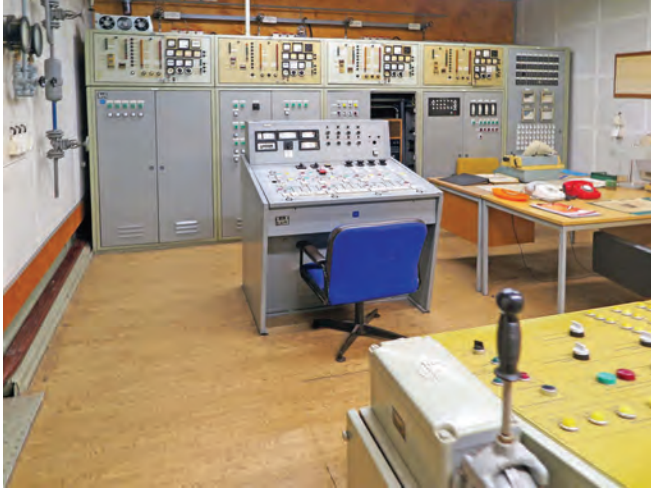
The Garzau bunker controller monitored and directed all aspects of the services from this console. Photo Clive Penfold
